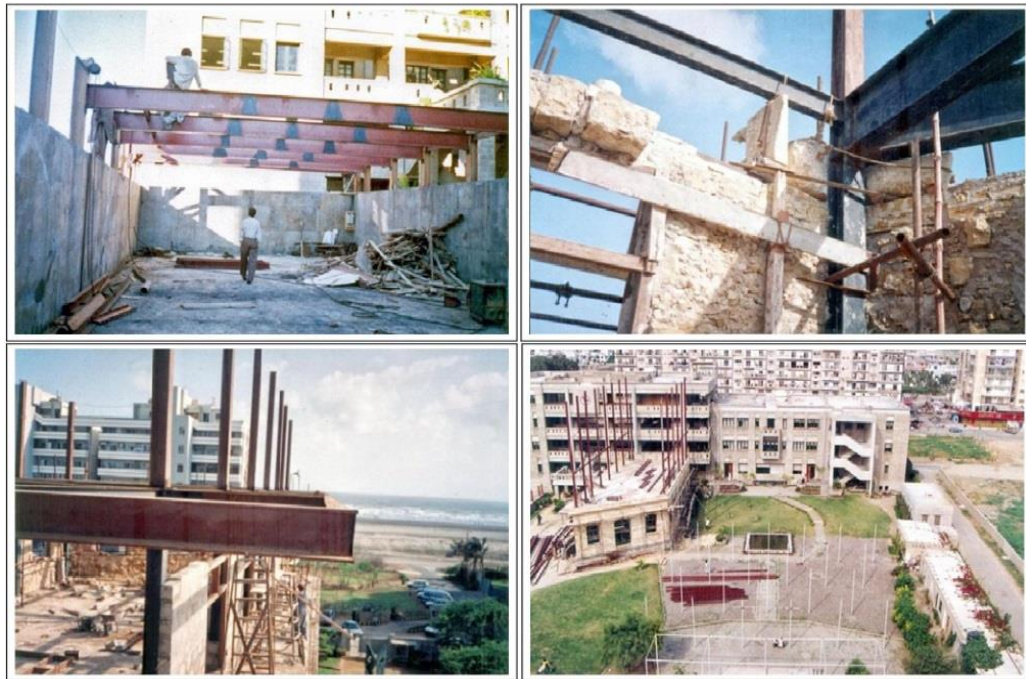
Figure 4: Laying of girders in the roofs of basement, 1 st floor, 2 nd floor and 3 rd floor for East wing
