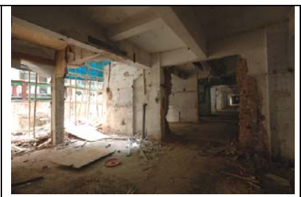
Figure 8: A temporary access way was formed inside the site for small machines for the handling of demolition materials
