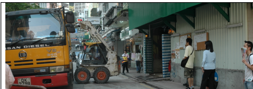
Figure 7: Work reality in congested urban environment. With the help of a banksman, debris was removed by a small loader making use of the public roadway with temporarily blocked traffic and pedestrians passing-by
