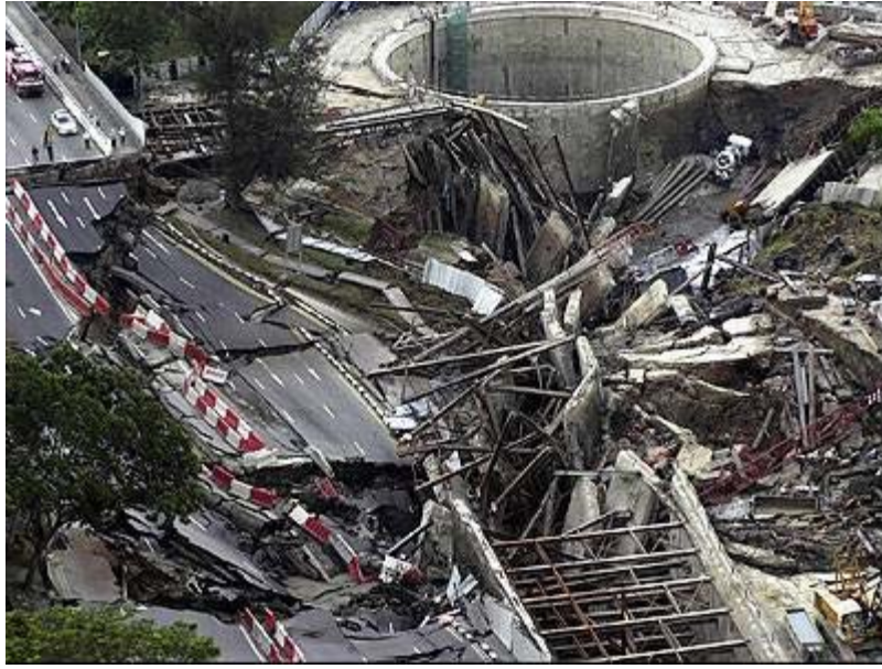
Figure 1: The site at Nicoll Highway after collapse
