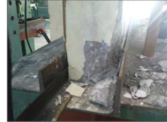
(h) Crushing failure at the bottom of wall panel
