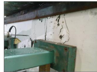
(g) Surface crack on wall panel
