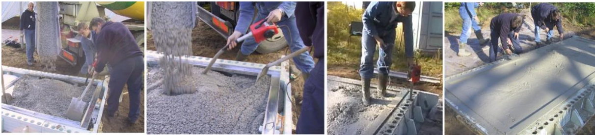
Figure 5: pouring concrete mortar on ground floor to fill foundation beams of pilot project
