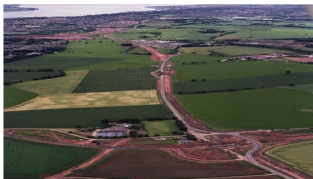
Picture 1: A92 PFI Road Project under Construction (Courtesy: MorganEST Rugby Office Archive)
