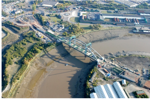
Picture 2: NSDR PFI Road Project and River Usk Bridge under Construction (Courtesy: MorganEST Rugby Office Archive)
