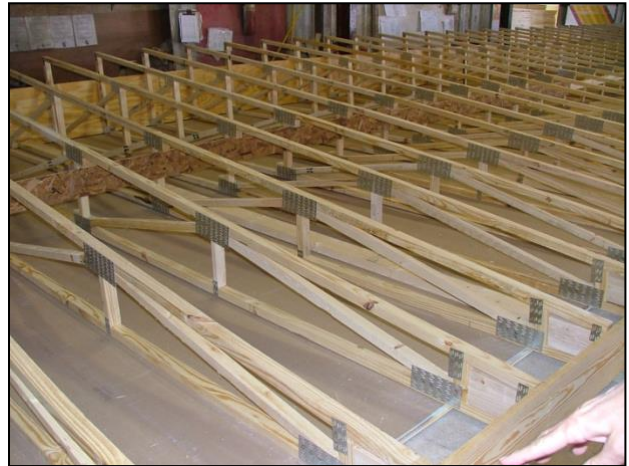
Figure 4: Roof trusses reduced from 24" o.c. to 16" o.c. and doubled at end walls. Drywall laminated to truss bottom chords (Draper, 2005)
