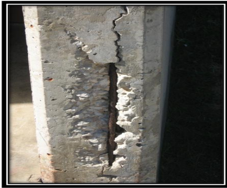
Figure 1: Spalling due to expansive forces of corroding reinforcement (Photo: H.J Duminy)
