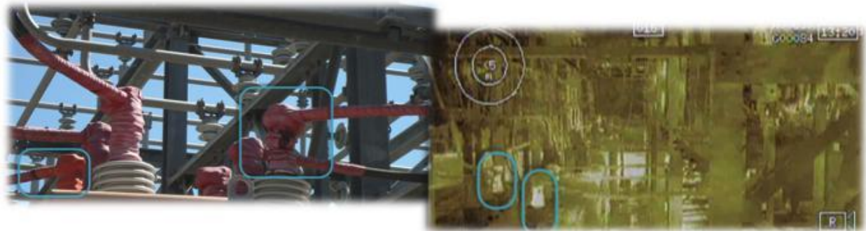
Figure 6: Infrared Substation Inspection
